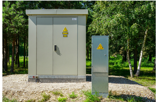
Electrical equipment located out of sight and within secured facilities
