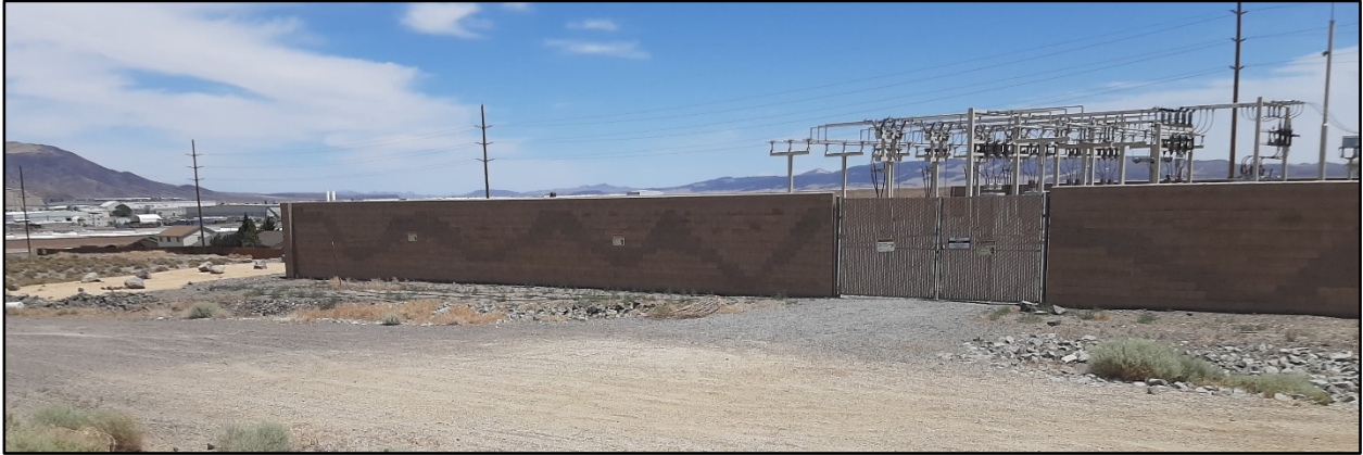
NV Energy substation panorama – view northeast
