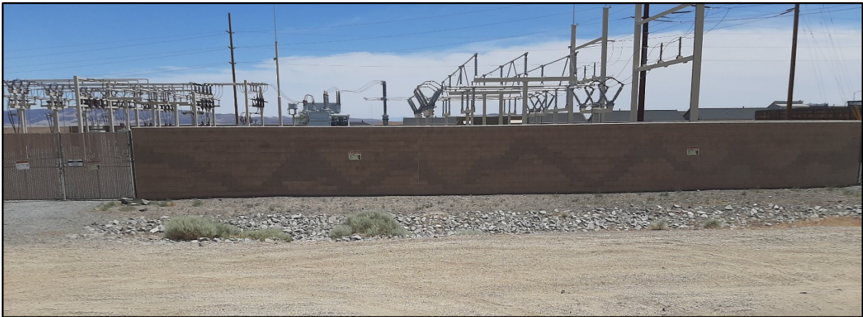
NV Energy substation panorama – view east
