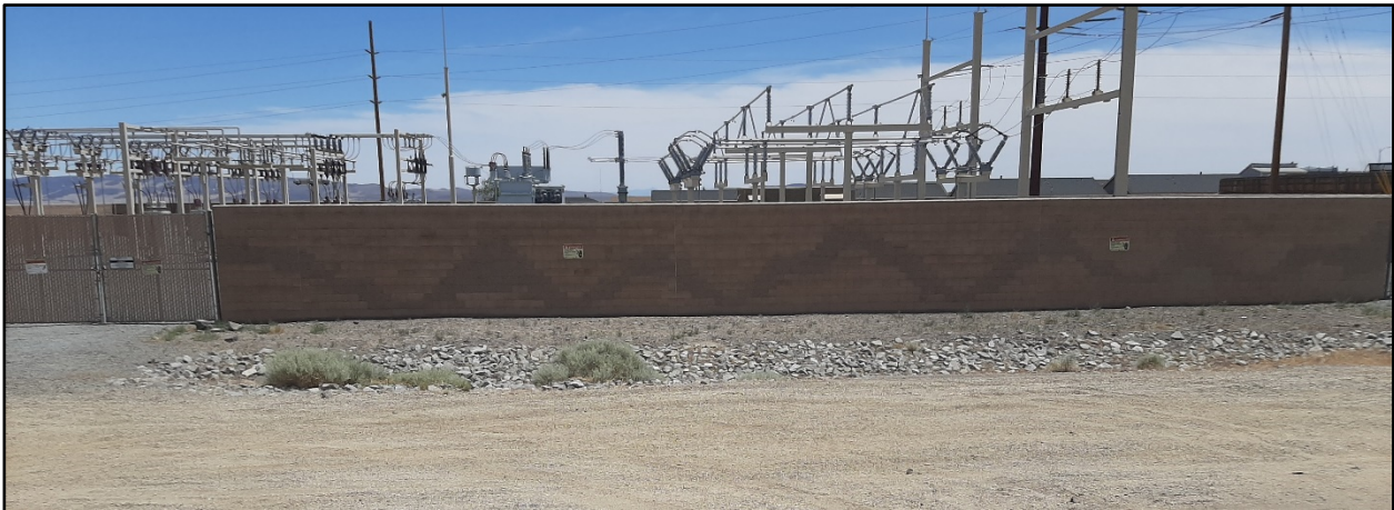
NV Energy substation panorama – view east
