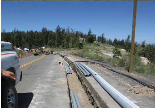
KMPUD Power Line Reliability Project
