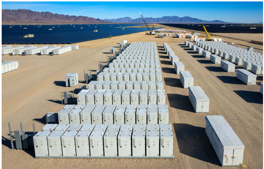
The Eland Solar-plus-Storage Center in Kern County, California (Credit: The Desert Photo/iStock/Getty Images Plus)
