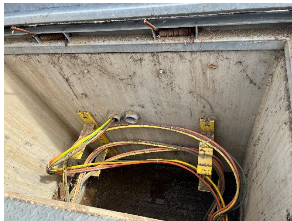
Figure 6.10 Handhole IMH-103, taken during site visit
