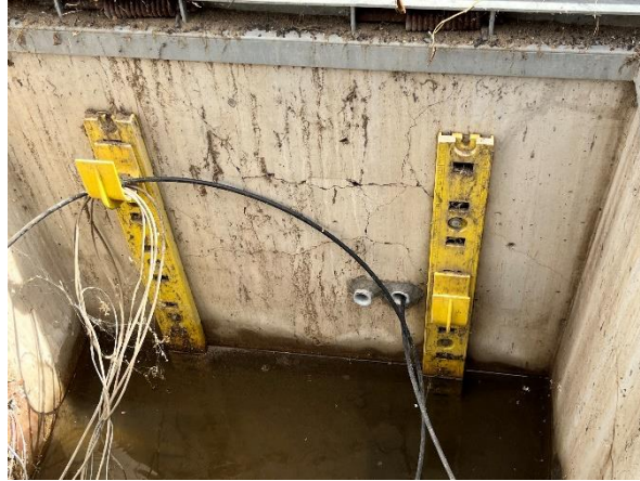
Figure 6.9 Handhole EMH-103, taken during site visit
