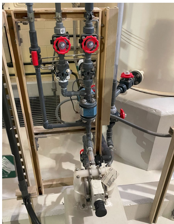
FIGURE 2-4: CAUSTIC SODA CIP FEED PUMP
