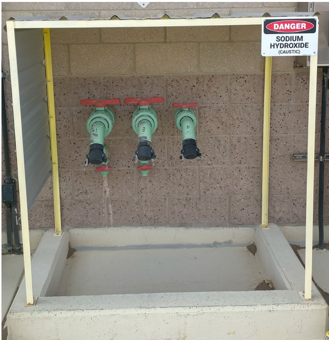
FIGURE 2-3: BULK CHEMICAL FILL STATION
